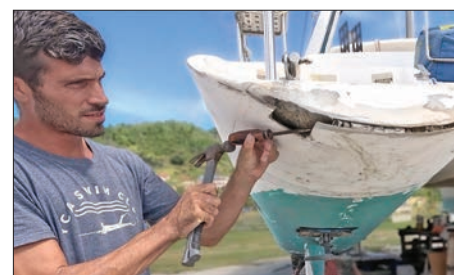
The boat needed extensive fiberglass repair. Fortunately, Huub found a professional boat-builder to help with the project.
