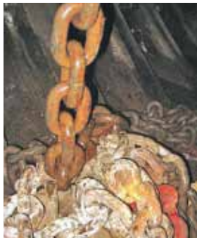
Chain locker distress.
