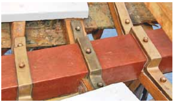
Some of Viveka's original oak timbers have been replaced with purple heart, and her original metal floors have been upgraded to solid bronze.
